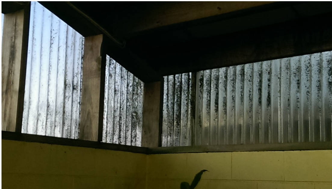
Picture 3: Pool Hall Internal Mould and Condensation
