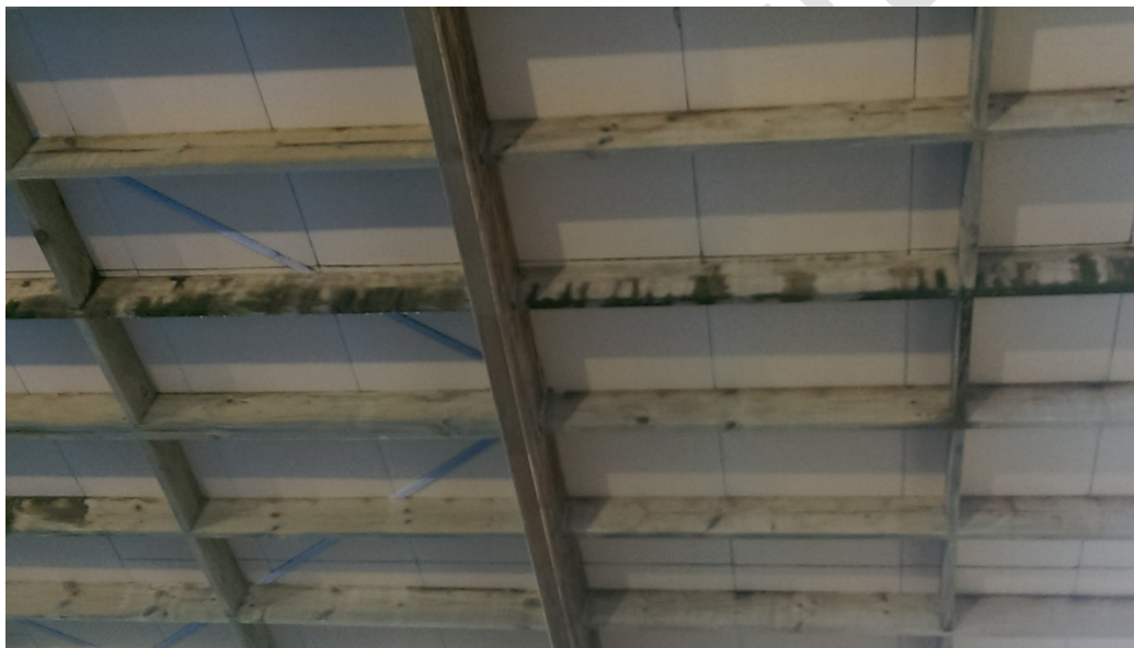
Picture 7: Pool Hall Breach through Joints in XPS and staining of timber
