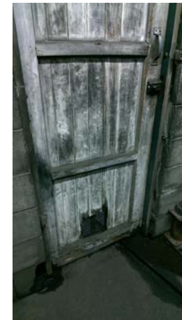
Door and ?? to Boiler
