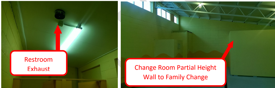
Picture 4: Restroom Exhaust & Change Room
