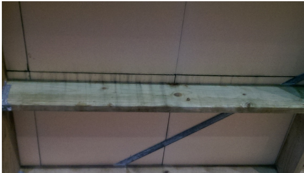
Picture 6: Pool Hall Breach through Joints in XPS
