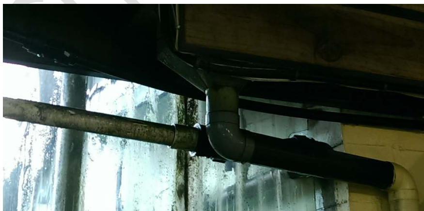
Picture 8: Pool Hall Internal Gutter
