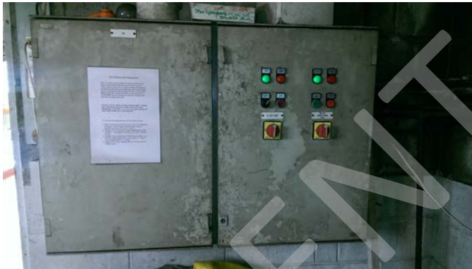
Main Switch Board
