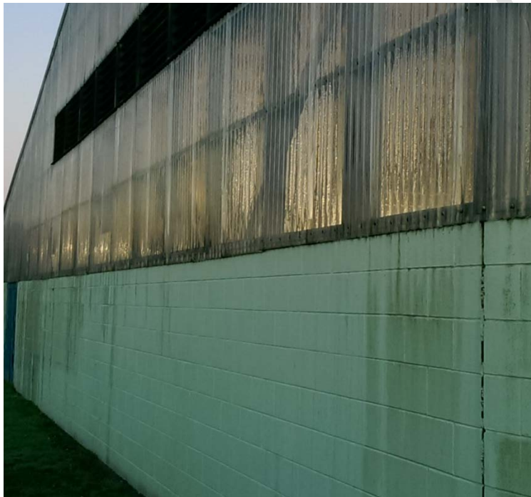
Picture 4: Pool Hall Mould and Condensation
