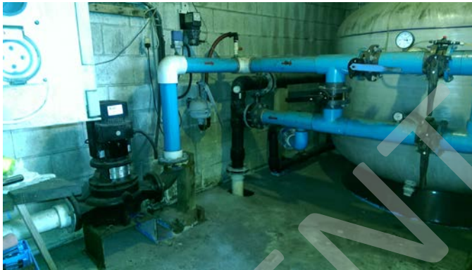
Pumps and Dosing
