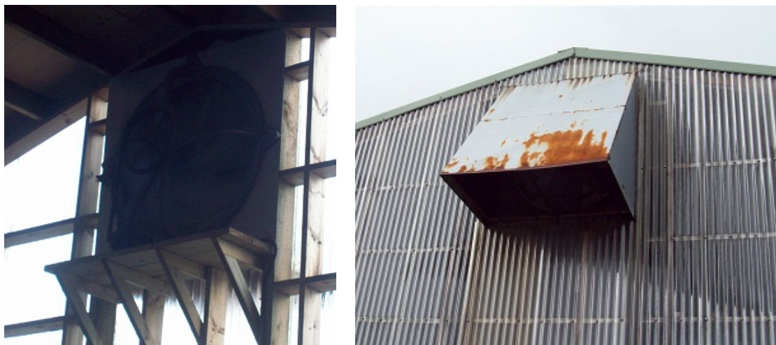
Picture 1: Pool Hall Exhaust Air Fan & Discharge Hood
